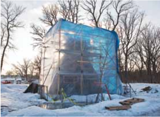
Kilmer Fireplace scaffolding was wrapped in plastic so masons could work through the winter
