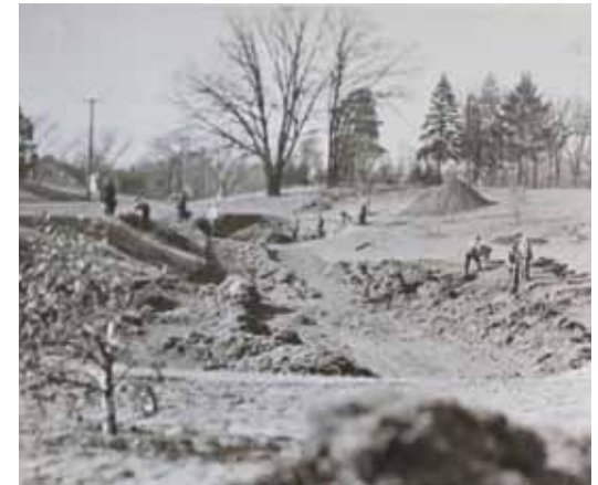
WPA labor built both the Kilmer Cascades (pictured) and the Kilmer Fireplace
